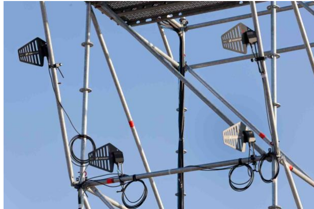
Four Spectera DAD antennas on a lighting tower
