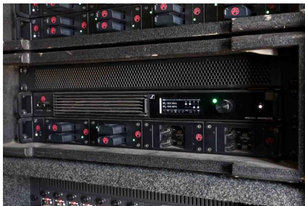
Spectera Base Station and L 6000 charging station
